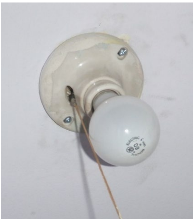
Figure 6: Example of an exposed incandescent lightbulb. Any kind of exposed bulb is a safety hazard and should be replaced by an enclosed light fixture.
