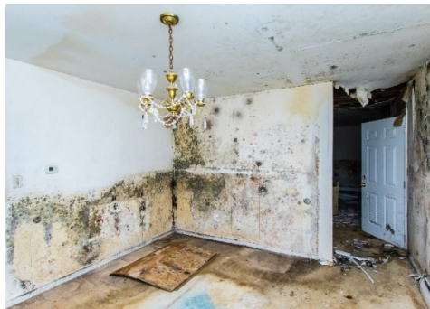
Figure 10: Mold on the walls of a house.
