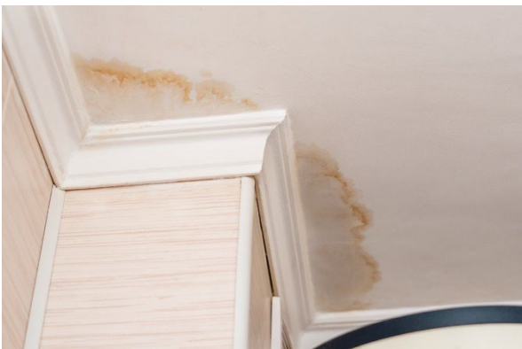
Figure 7: Example of water stains in the ceiling.
