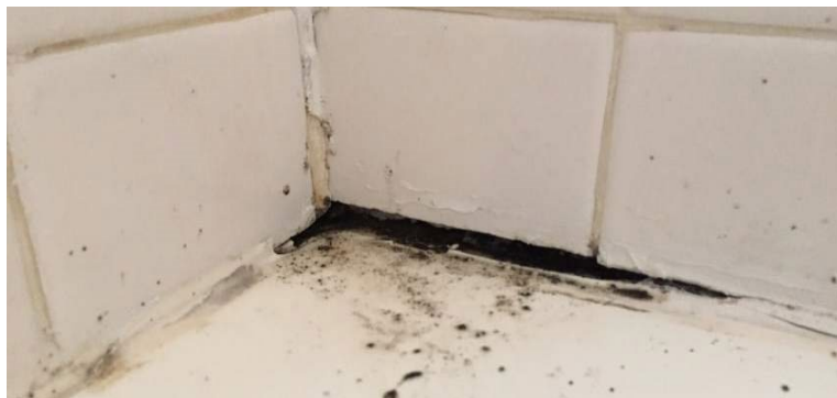
Figure 11: Mold growth in a shower.
