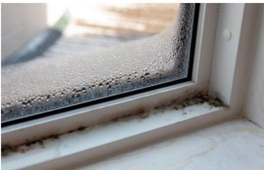
Figure 9: Mold growing around a windowsill.
