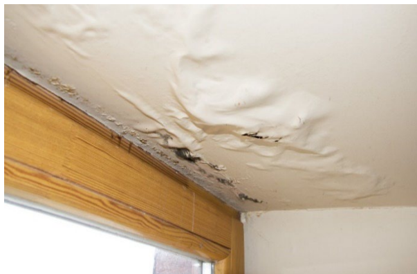
Figure 8: Example of bubbling paint caused by water damage.
