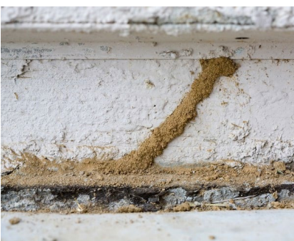
Figure 16: Termite tubes on the side of a house
