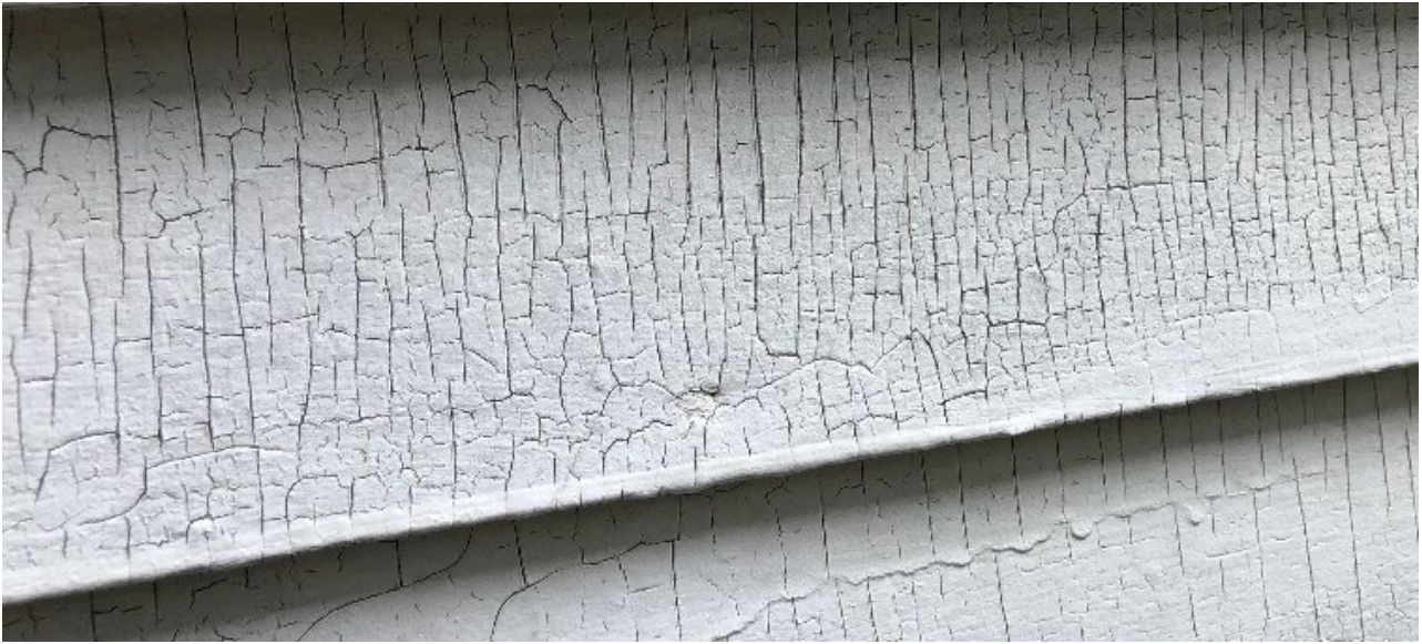
Figure 1: "Alligatoring" lead paint. This distinct pattern is a result of the oil base in lead paint. Not all oil-based paints are lead paints, but alligatoring is a good indicator of lead paint in a residence.
